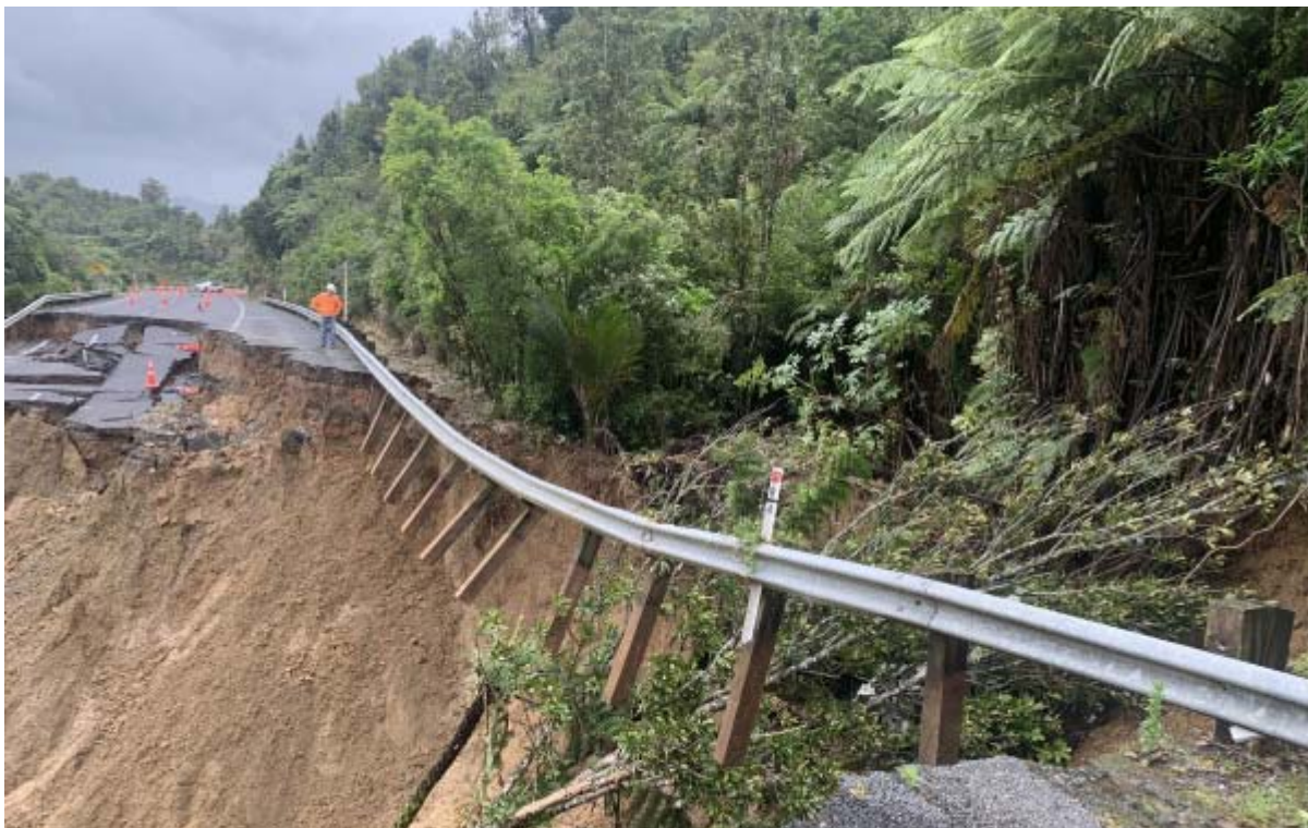
Collapse of road at summit of State Highway 25A which links Tairua with Thames. Photo: Waka Kotahi.
