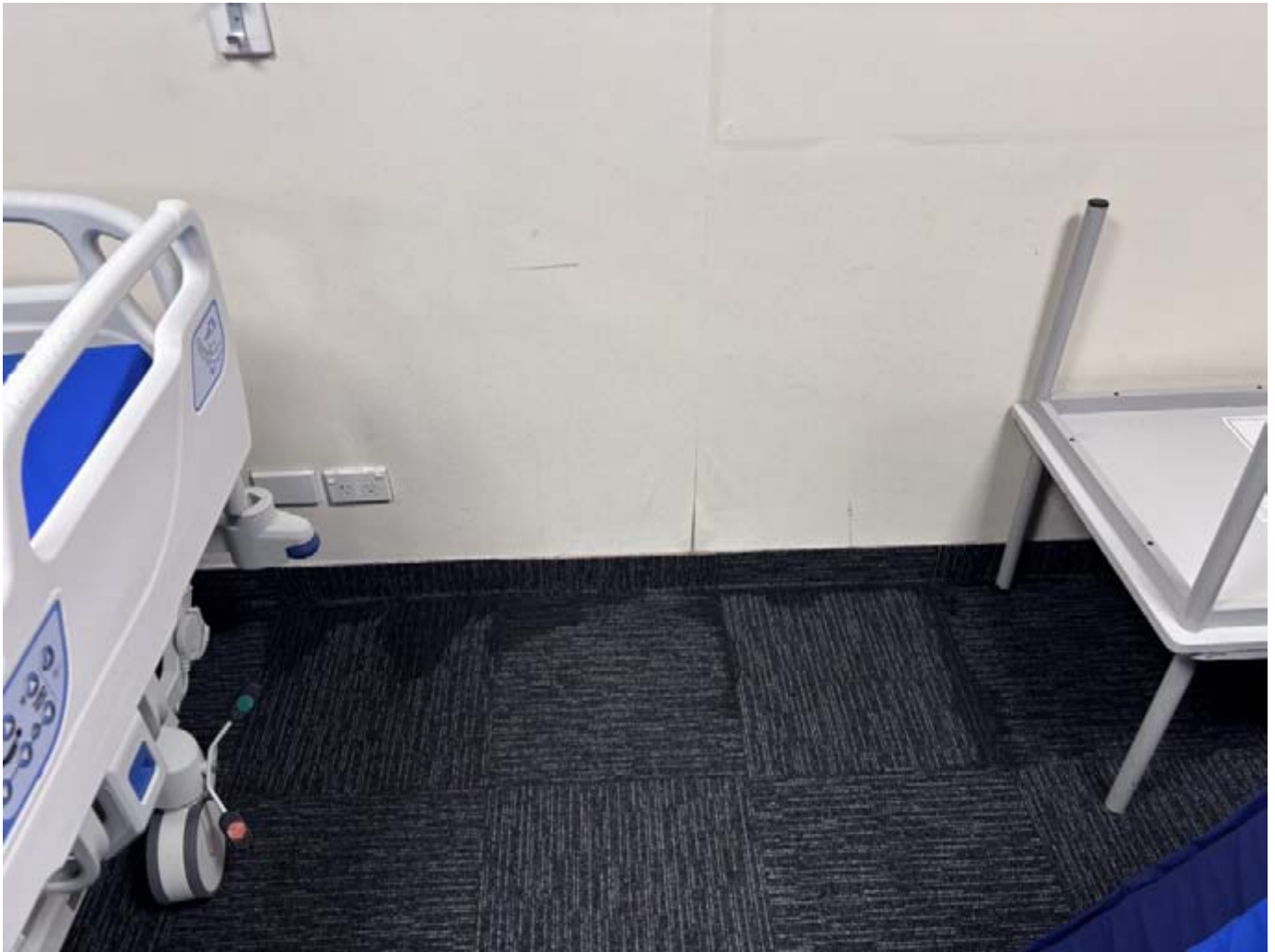
A patient bed next to a leak in the floor and lower wall at Hutt Hospital.
