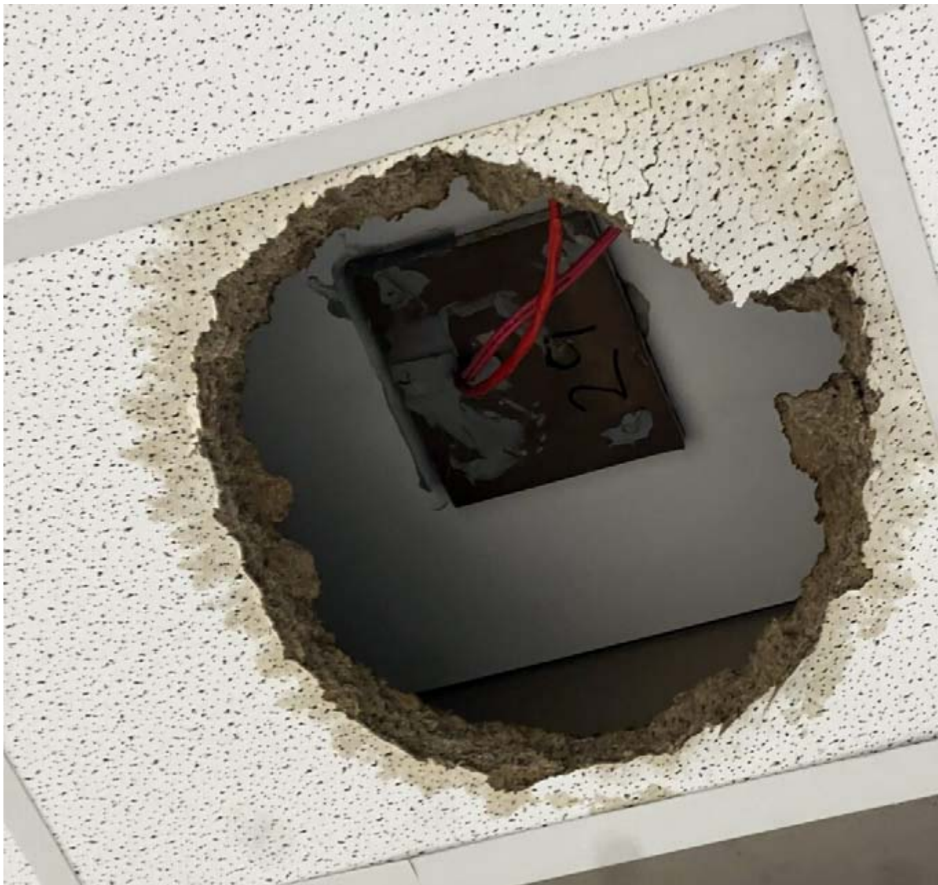
A view of the water-damaged ceiling at Hutt Hospital.
