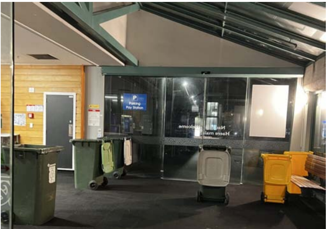
Wheelie bins used to catch water at the main entrance to Hutt Hospital.
