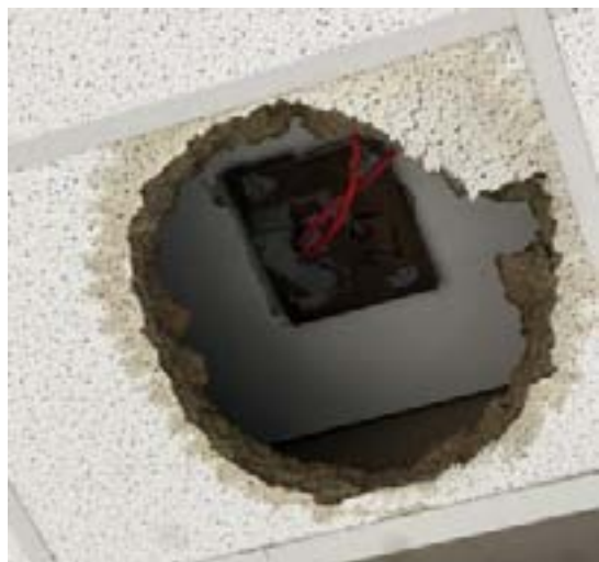
A soggy ceiling panel leaving a void at Hutt Hospital.
